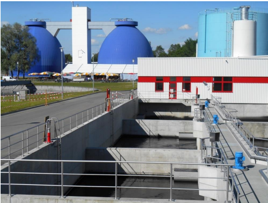
At the Langwiese wastewater treatment plant, a basin with activated carbon has been added as a fourth stage of purification. Photo: Rita Triebkorn
