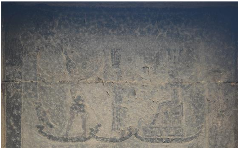
Before: A ceiling covered in thousands of years' worth of dust and soot.
